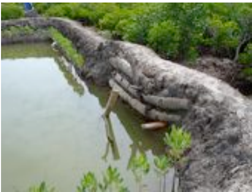
Figure 2. A pond at Majaoni showing stand pipe for draining the pond and overflow pipes to relieve the pond of extra water at spring high tides and increase water exchange in the culture ponds.
