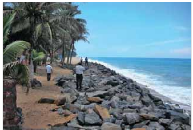
Revetments on Ullal Beach, Mangalore, India provide protection to life and property during the southwest monsoons
