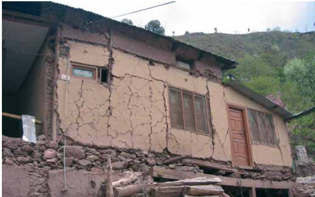
Destroyed house in Saidpur: Karen Sudmeier-Reiux, 2007
