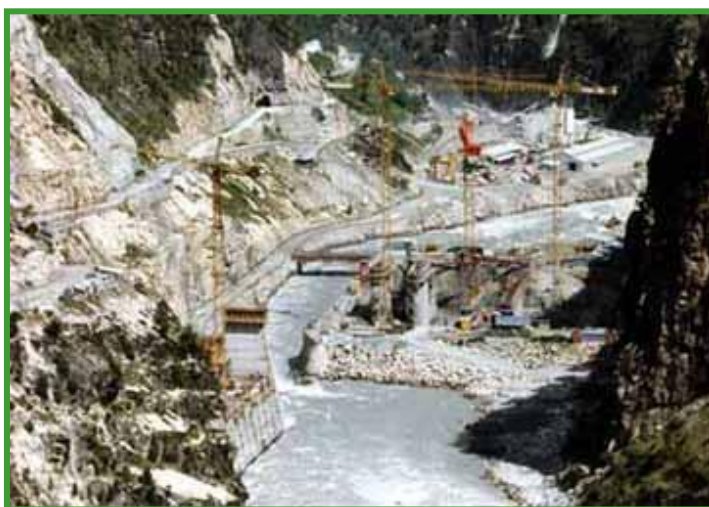
Figure 16. Dul Hasti hydro-power project on Chenab
